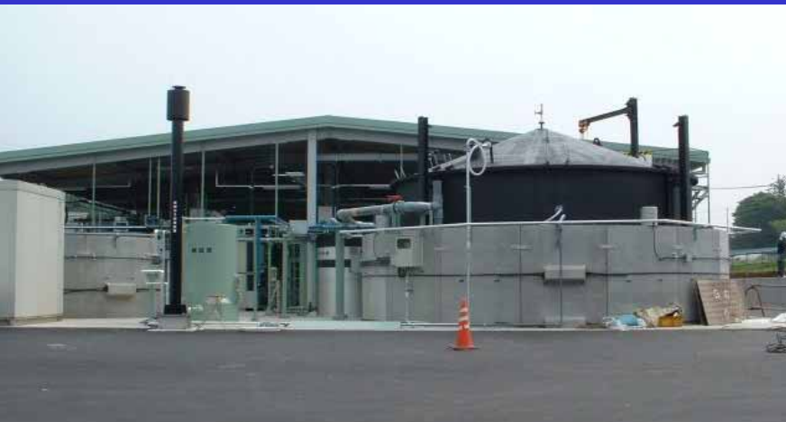
Methane Fermentation Tank
