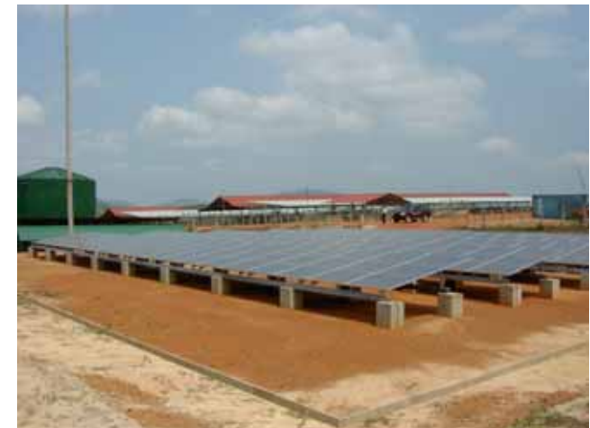
PV panels (24m X 29m )
