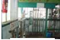
Operator's Control Room
