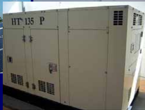
Generator 135 kW using Diesel+ Biodiesel (up to 50%)
