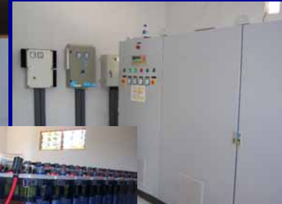
Control unit for hybrid system (converter DC=AC)
