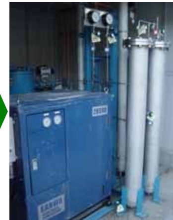
Desulfurization tower CO 2 removal tower
