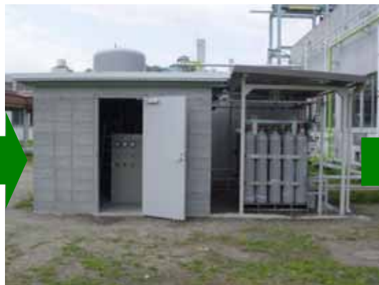
Compressor & Gas holder
