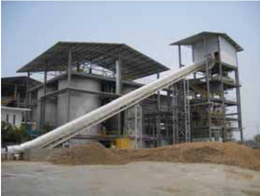
Bagasse Feed Conveyor
